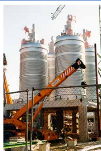
4 reactors 110 m 3 3 stages of GlasLock ® agitators
